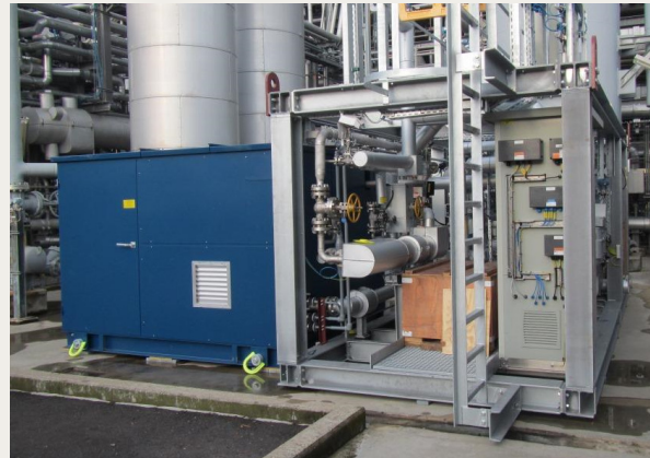
Figure 7: Membrane side stream unit
